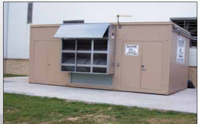
The DirectAIR® Compressed Air Facility
