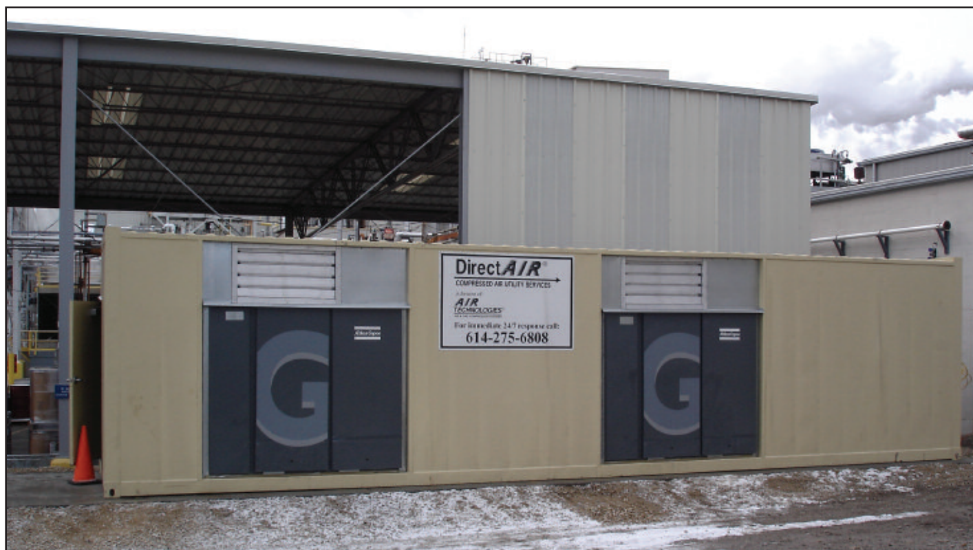
DirectAIR Installation With Atlas Copco Compressors
